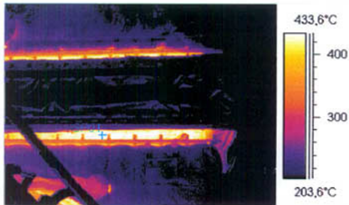
Flange and bolt temperatures in an exhaust duct, measured by thermograph.
