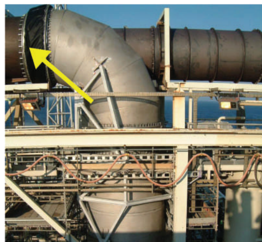
Thermobolt installed on an LM2500 Exhaust Duct.
